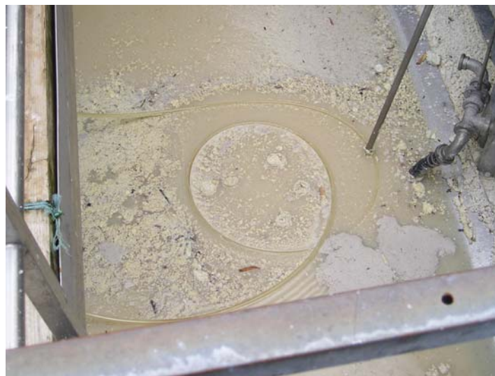
The thin fat layer is destroyed by the oil collector tube and fat sticks to the oil collector tube
